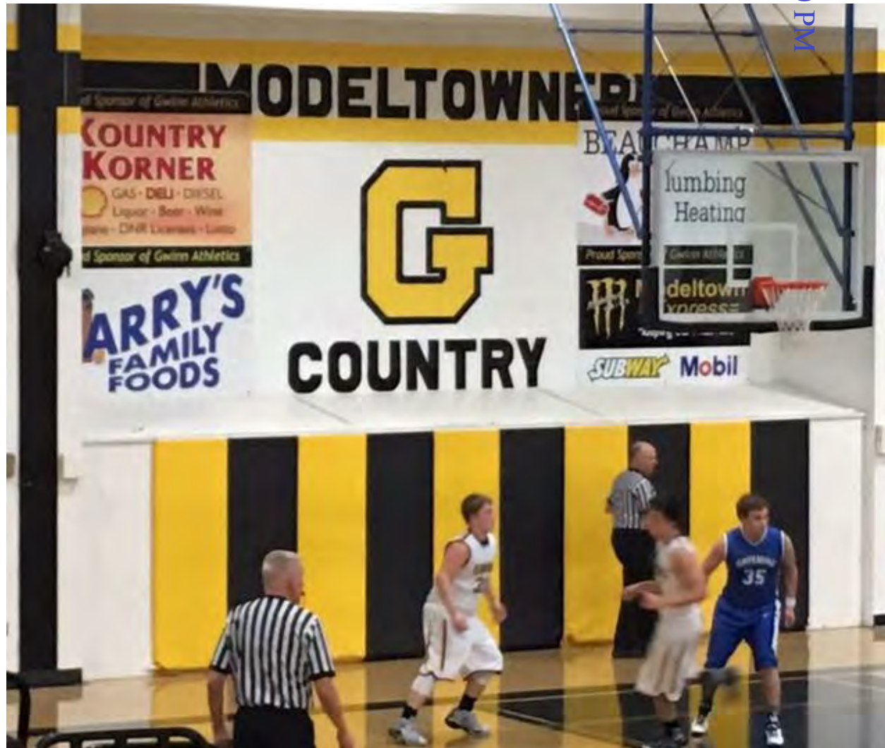
Figure 4 - This photo, taken between 2010 and 2015, shows the padded safety enclosure installed as intended for the safety of athletes, students and other members of the public.
