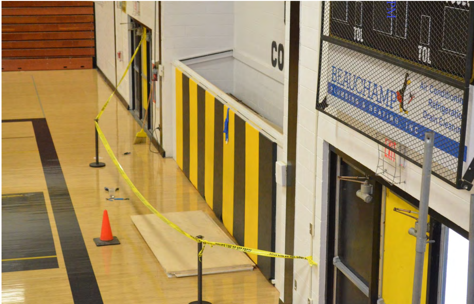
Figure 5 - Immediately following the tragic incident on September 3, 2015, the wall panels were installed and secured to the building. The photo was taken as part of the police investigation. The area around the enclosure was cordoned off during the installation process. The plywood sheets on the floor form the ceiling or cover for the enclosure. See Figure 4 , above.
